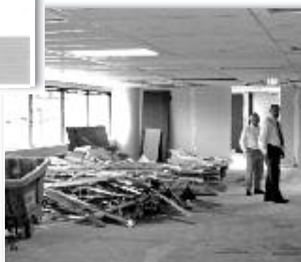
Colorado Nonprofit Association completed the remodel/expansion of its current 455 Sherman St office suite simultaneous with the rebranding, to enhance the professional appearance of the office and to accommodate staff growth. Lew Bakkeemo (left), receptionist, and Charley Shimanski, president & CEO at the time, tour the office demolition in the photo below.
